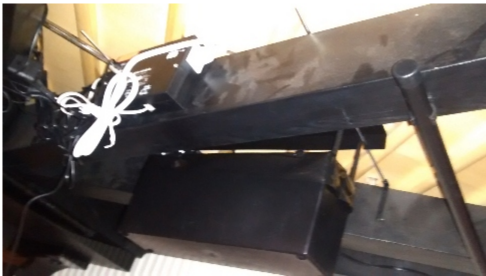
On the right of the photo is the secondary heater at the tail of the piano; in the middle is the water tank; and top left is the control unit.
